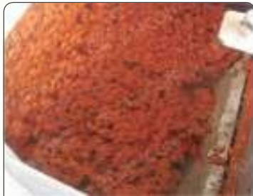
2 Flocculation Tank 絮凝槽
