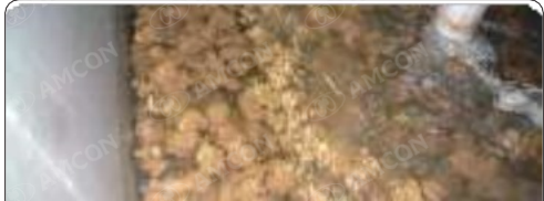
3 Flocculation Tank 絮凝槽
